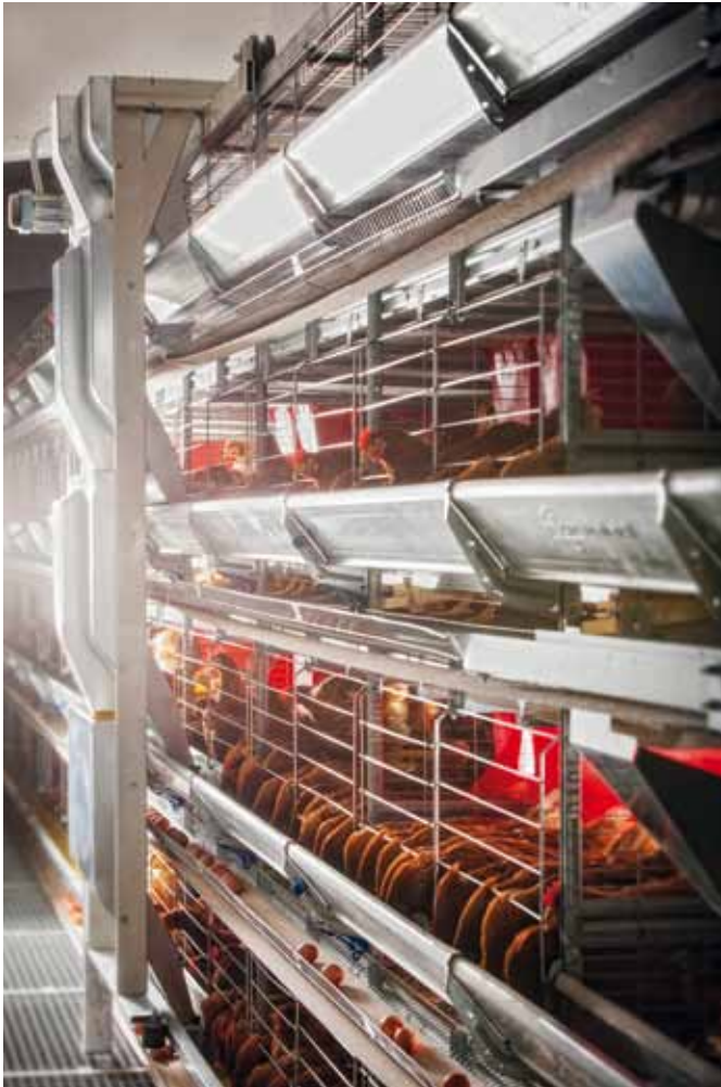
> Corridor with feed trolley
